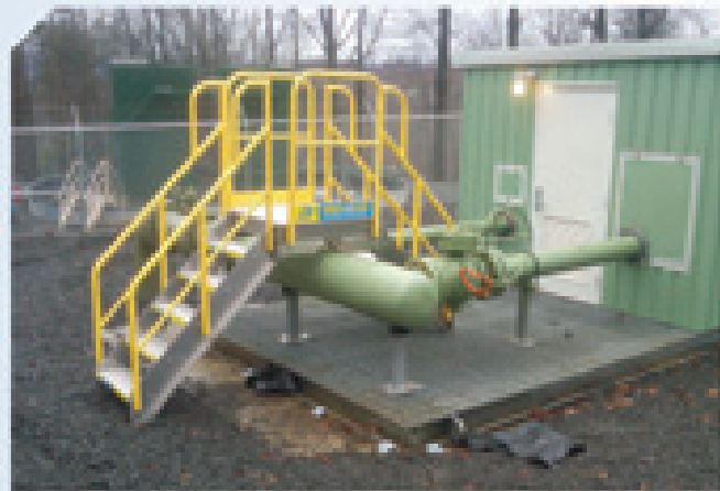
Pump station access was an afterthought.
